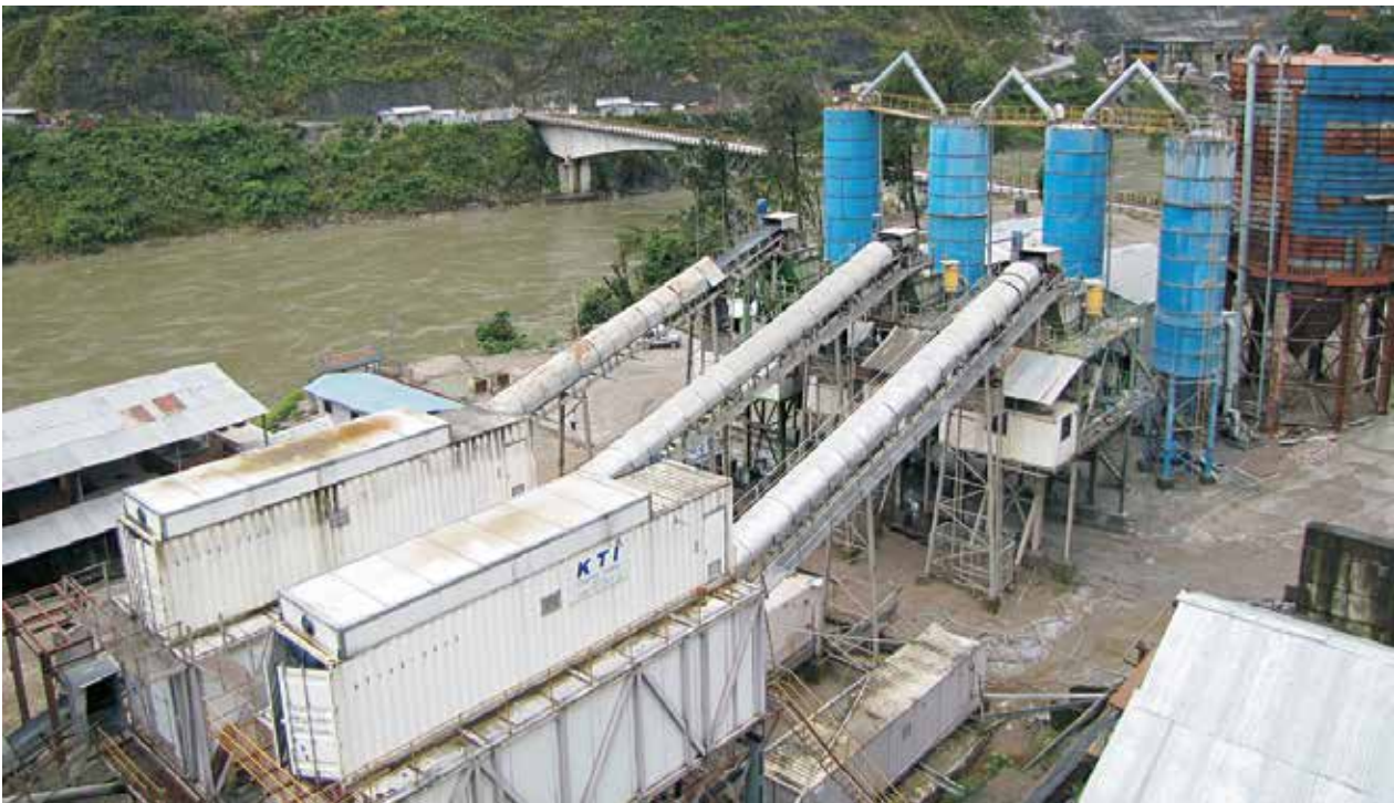
The H6 plant at Subansiri in DAM concrete that set record in PQC production (6020 cu.m in 1 day)
