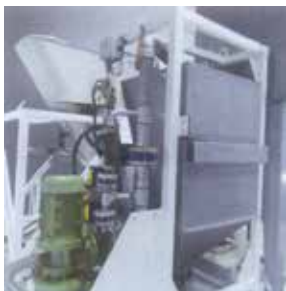
Water weighing system with discharge pump for pressurised feeding of water into the mixer .
